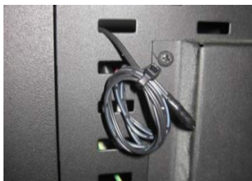
Figure 22 - Room temperature probe
